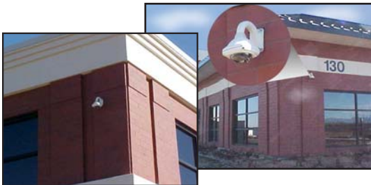
The WP7 Warrior Pan/Tilt was chosen for its vandal and weather resistance qualities. Part of the 32 unit installation at Littleton includes these WP7's guarding the exterior of the building.
