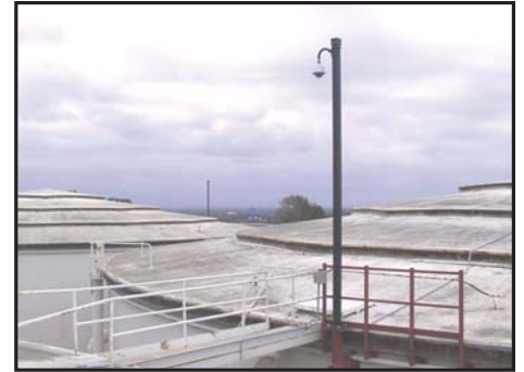
Sitting atop the 33 foot tall tanks, the PV16 allows the camera to have a clear view of other tanks and the rest of the property. Access for servicing is easy using the tank stairway.
