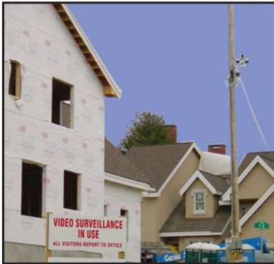
A clear warning is posted that the Videolarm PT55 is on guard as construction continues on Eastland Townhouses
